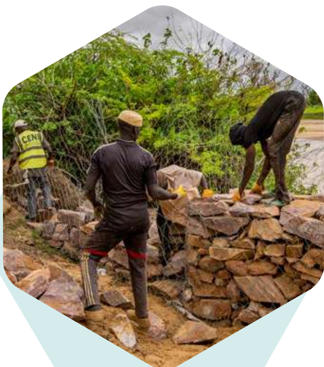
Construction of a flood-protection dam in the cultivation area of Maradi, Niger. © FAO
