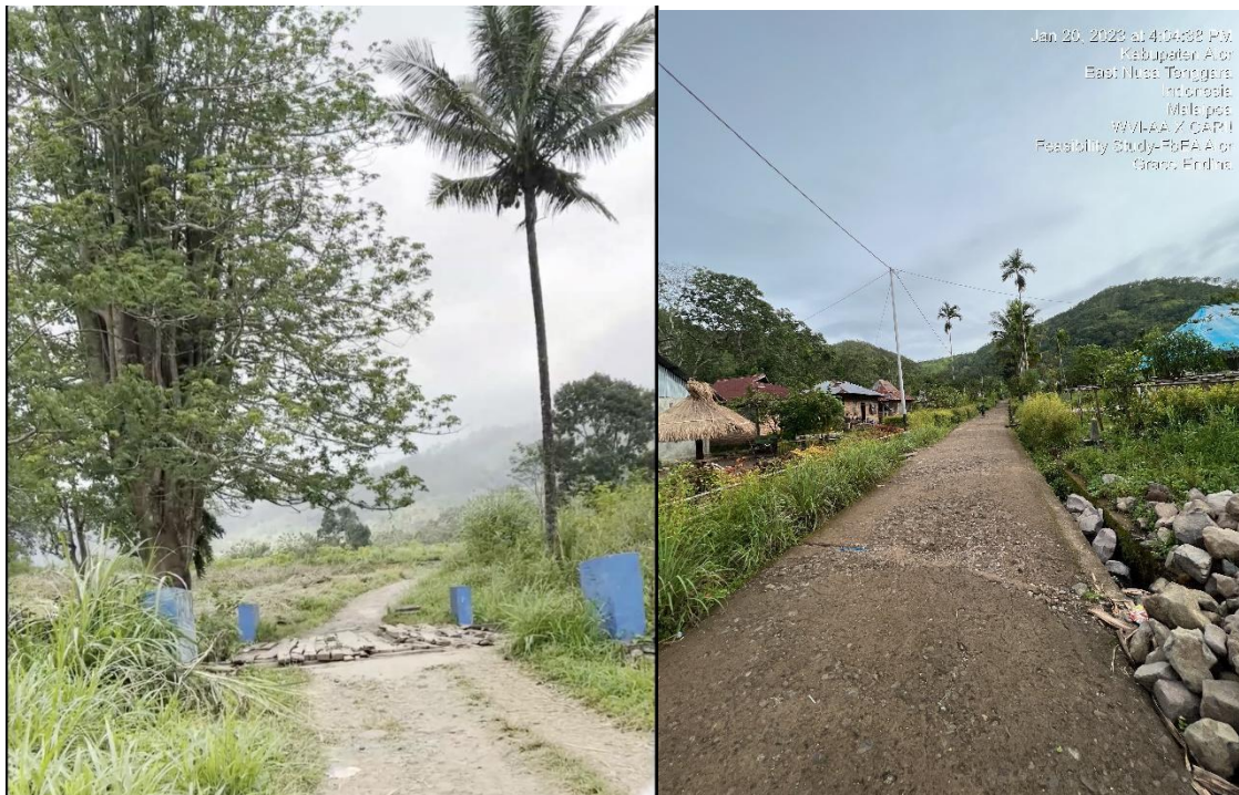
Figure 48 Heavily damaged road with a temporary bridge in Malaipea village (left); unpaved road in Welai Selatan village (right)
