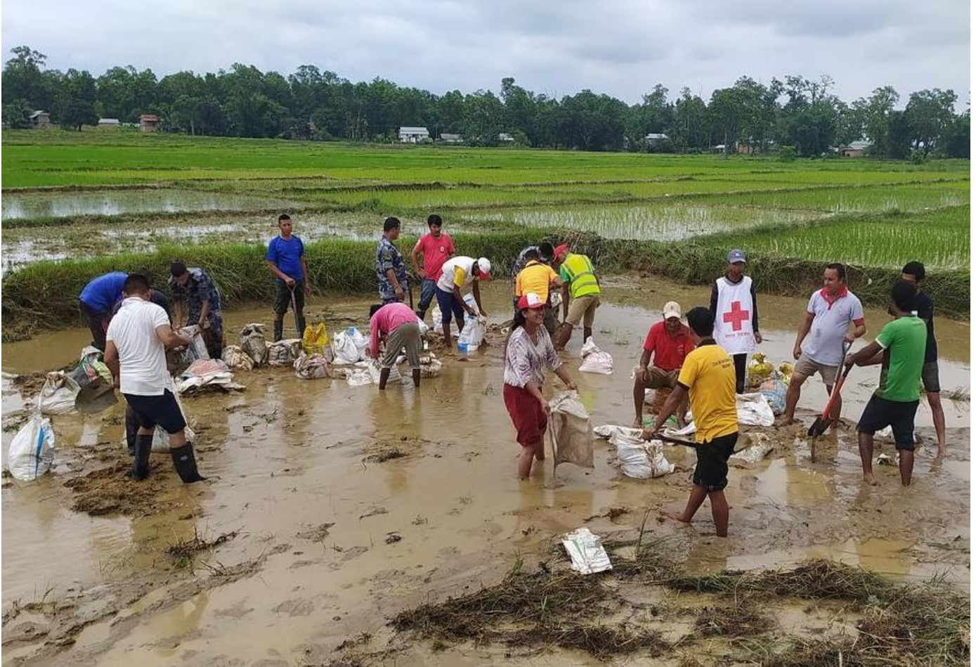
NRCS volunteers and local people mobilised to strengthen embankments, preventing floodwater from entering the settlements. (Photo: Nepal Red Cross Society)
