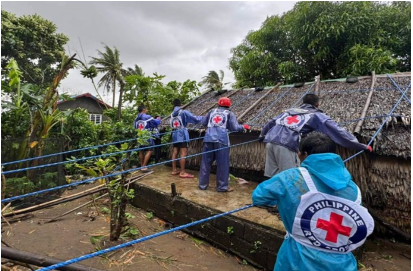
Installation of Shelter Strengthening Kits in Villa Leonora, Buguey, Cagayan as part of Typhoon Marce Activation on 6 November 2024. (Photo: PRC)
