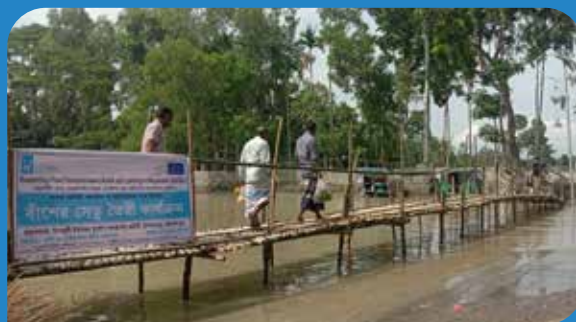
SUFAL Project supported the building of temporary walkways a week to a few days ahead of the floods to ensure uninterrupted mobility of people living in low-lying areas around Kulkandi union of Jamalpur district. Without this, people would need to travel a distance of 2 kilometres to reach the other side of the canal.
