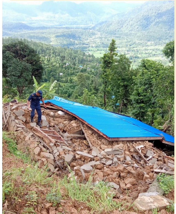
A house collapsed by landslide in Gurbhakot. Image: Dilli Pun
